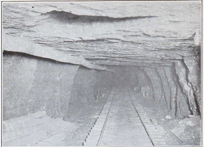
A 500-foot Line of 8-Inch Flexoid Tubing suspended from the roof.
